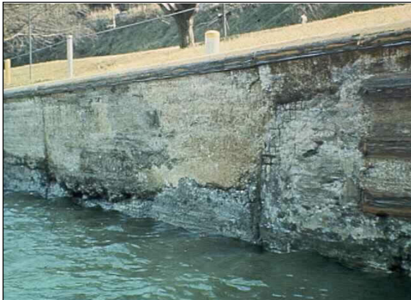
Crumbling lock wall, Lower Mon 3, opened in 1907
